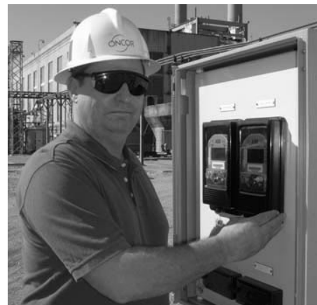
David Welch, Oncor Transmission Metering Specialist, demonstrates the installation of the new EPS Meters.
